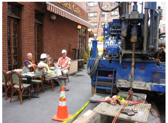
Lunch by the drill rig during testing for the 2nd Ave. subway, New York City, 2005 (Photo by Thomas Doe)
