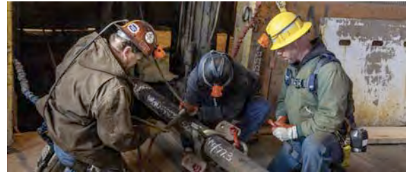
Figure 6: Rope Technician Rick Tinnell and Infrastructure Technicians Jason Graves and Pat Urbaniak prep a 33-foot pump motor to be lowered down to the Yates Shaft
