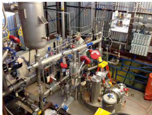
Figure 2: LBNE prototype cryogenic system
