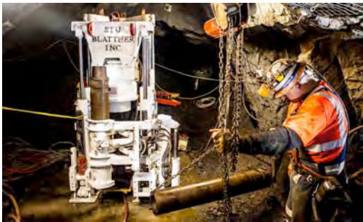
Figure 5: A crew from Stu Blattner Inc. changes a pipe on a drilling rig at the 1700 Level. The cylinder in the foreground is a button bit cutter. The reamer uses four of these cutters and is pulled up or back reamed to widen the pilot drill hole, creating a raise.
