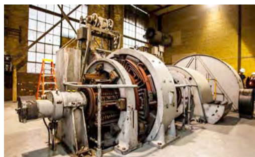
Figure 4: The motor-generator set that converts AC power to DC power to operate the hoist.
