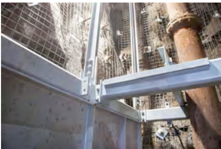
Figure 8: A bearing beam in concrete, with new rock bolts and ground support. Pump column at right
