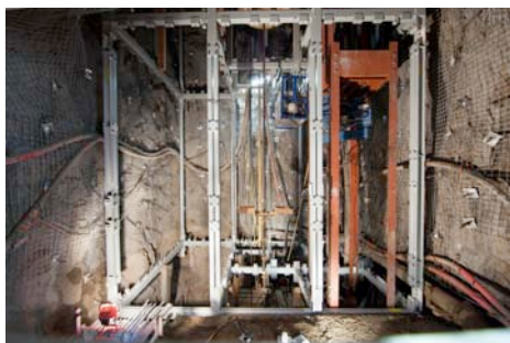
Figure 5: The Ross Shaft as seen from the station at the 300 Level. Suspended at the upper corner, is a blue Sky Climber lift.
