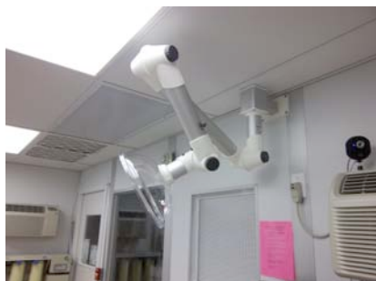
Figure 4: The newly installed Snorkel, with adjustable arm to move it out of the way when not in use
