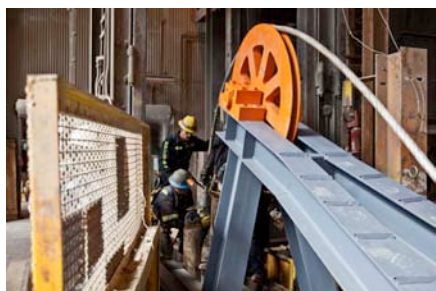
Figure 5: Infrastructure technicians Bill Heisinger (kneeling) and Trevor Ray attach a "cheese weight" to the end of the steel-wire rope to stabilize it
