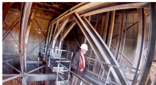
Figure 4: Project Engineer Mike Johnson, who is overseeing the rope-dog project, inspects the top of the rope-dog tower. Photo by Matt Kapust is a composite of two frames from a time-lapse video sequence.
