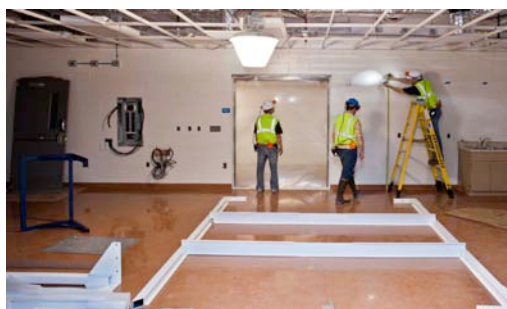
Figure 3: Steve Elliott (at right, on ladder) takes a measurement to install framework for a soft-wall clean room inside the MAJORANA assembly area
