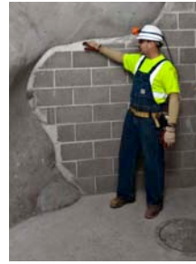
Figure 7: Rick Labahn points out the tight seam between a block wall and a shotcreted rock wall in the MAJORANA DEMONSTRATOR laboratory
