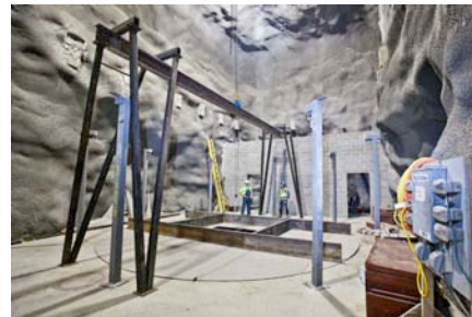
Figure 4: Project Engineer Rick Labahn (right) and Education and Outreach Director Ben Saylor inspect the temporary gantry at Davis Campus
