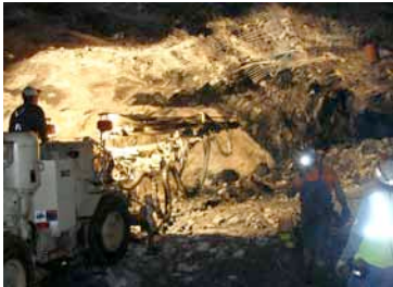
Figure 3: Mike Oates (left) operates jumbo drill at 4850 Level. Lighter colored rock in front of the jumbo is rhyolite.
