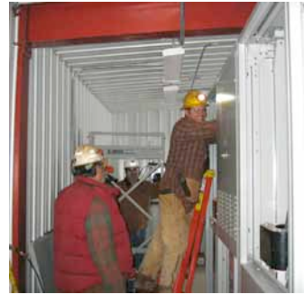
Figure 8: Facilities Techs Mark Javersak (left), Jason Rath (ladder) and Engineering Director Rick Labahn, working on Oro Hondo phase swap
