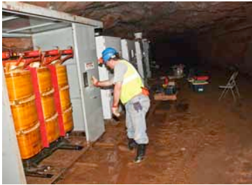
Figure 6: Mike Heinrich of Hydro Resources checks out the transformer. Steel wall in background is 6 Winze.
