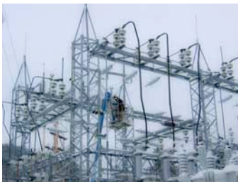
Figure 7: Karl Besler of Besler Inc. at the 69kV Oro Hondo substation
